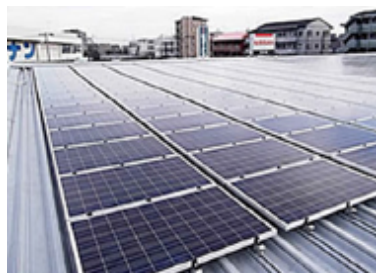
Solar panels installed on the roof of a Kanagawa Nissan dealership. Power from the panels is supplied to dealerships through the Nissan PPS system.
