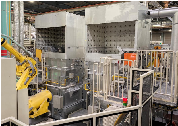
Fig.15 Appearance of Independent melting furnace for each casting machine
