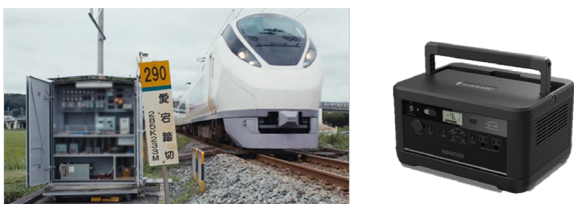
(a) Emergency power supply (b) Portable battery
